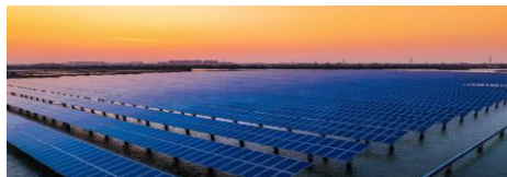
DVC 35 MW Solar Project
